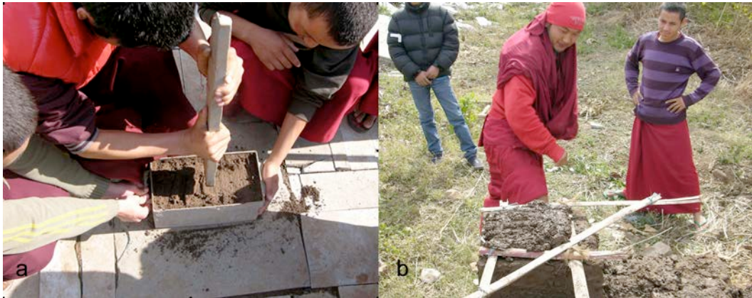
Fig. 6 – Dehradun, India, the winter workshop: (a) the production of different pakbu and; (b) the improved corner joint of the walls due to a simple structure constituted by a band with two timbers in parallel and diagonal members for bracing at corners (credits: Mauro Bertagnin, 2011)
